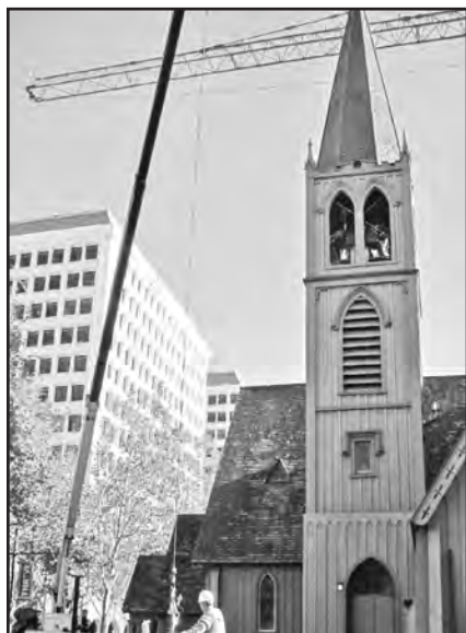
Bill Meeks, Meeks, Watson & Co., and Roger Lobbes, Trinity Cathedral, prepare to hoist a bell
